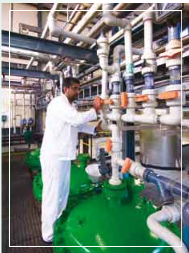
The downstream plants performed well throughout the year, with record production being achieved at the newly expanded lactulose plant at Merebank.
